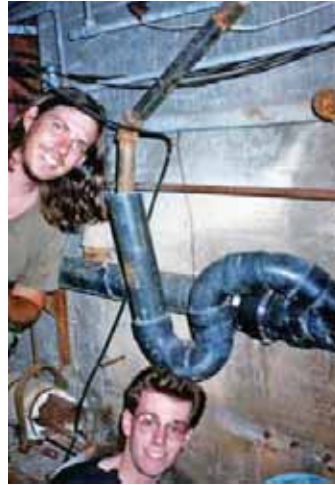
William "Schlake" Colburn and Operative Sushi show off some of the landscape of the Workman Center tunnels. Note the bizarre twisted pipe in the center, the rusted-out pipe at the bottom, and the fiber optic cable immediately in front of Schlake's head.
